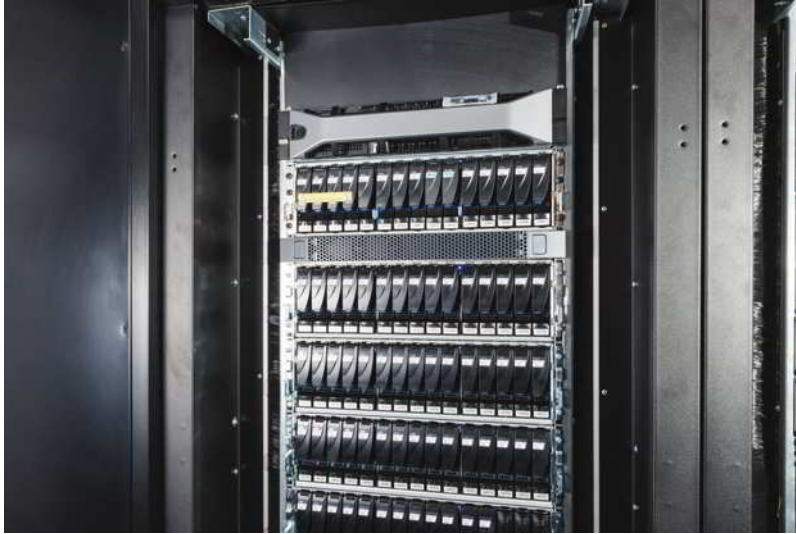
Figure 11.14 A storage array.
